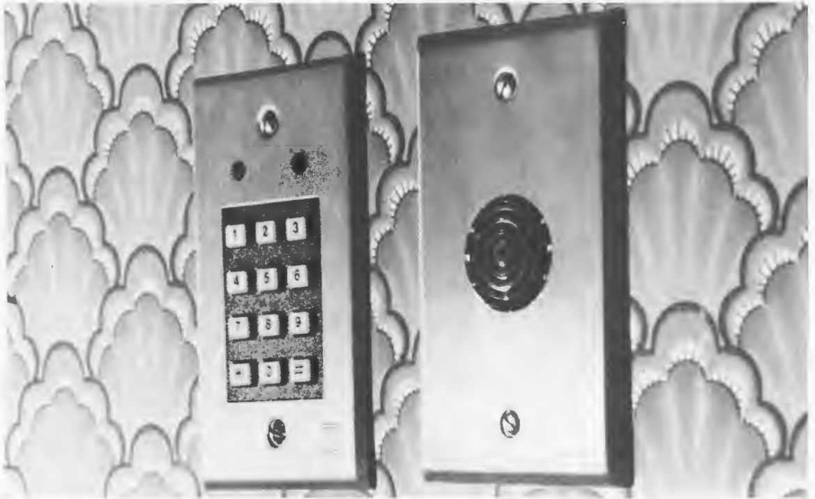
Fig. 18-13. Keypad and buzzer located in first floor hall.
