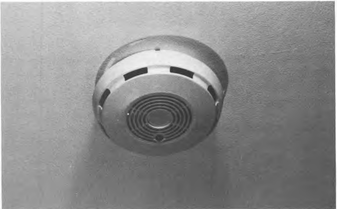
Fig. 18-19. A smoke detector located in the second floor hall constantly monitors for traces of fire.
