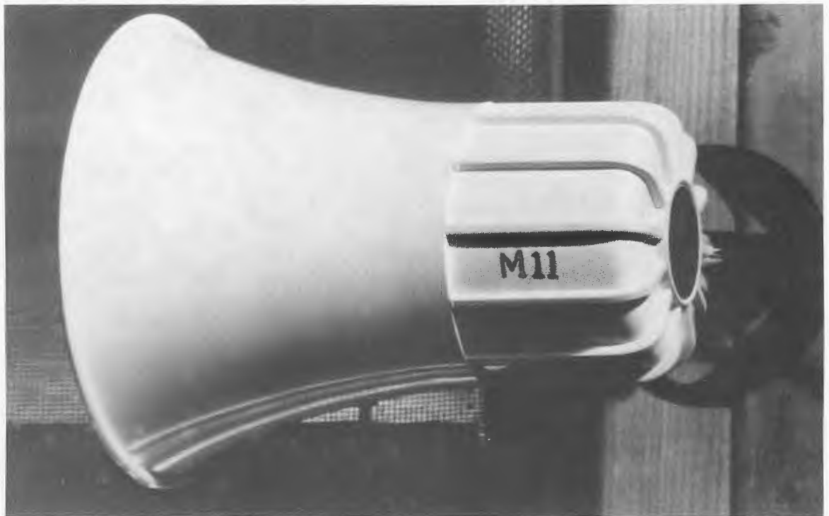
Fig. 18-24. Located at the attic vents is a siren to signal the neighborhood of an emergency.
