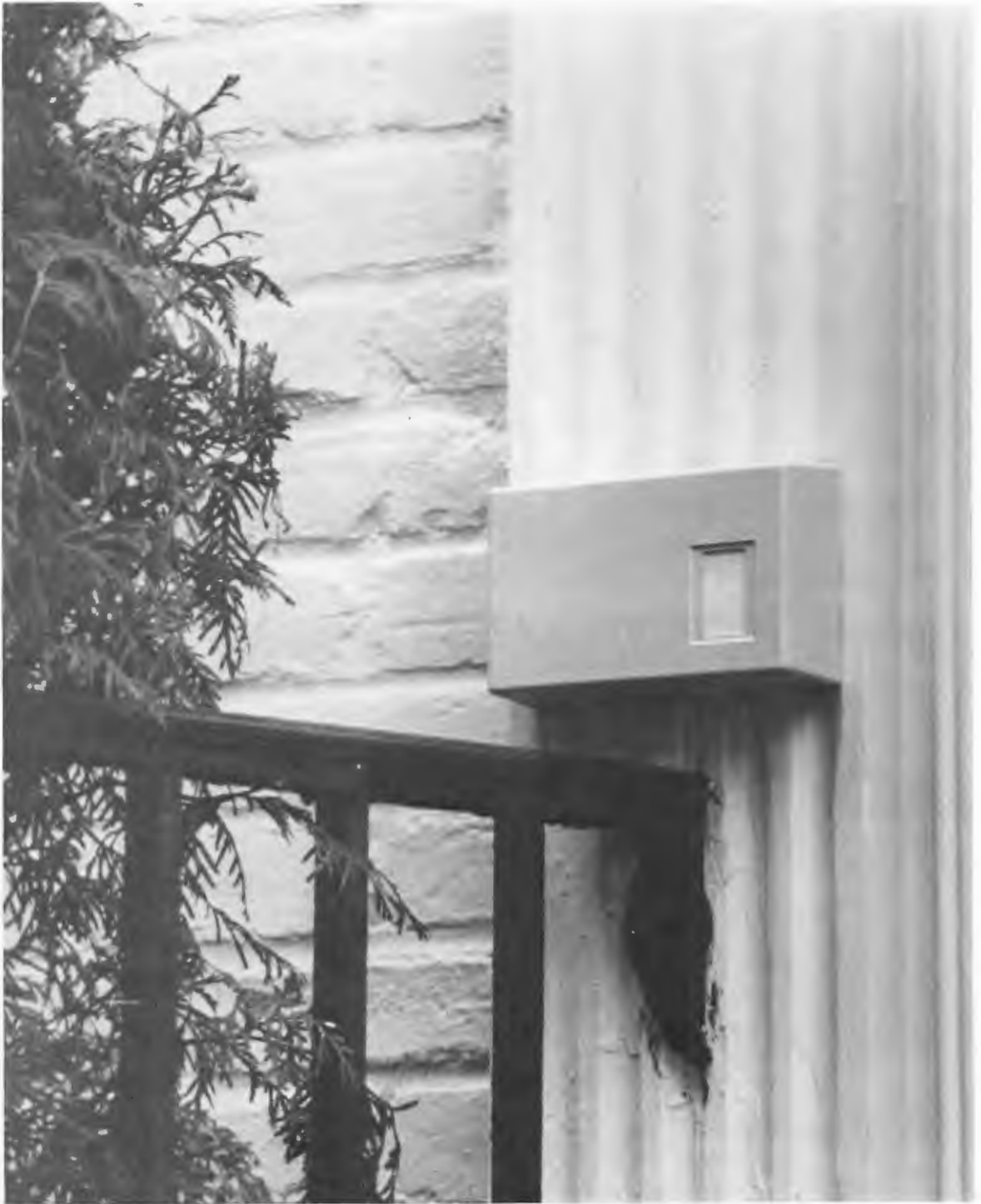
Fig. 18-11. Motion detector on outside of house takes note of visitors approaching front door.
